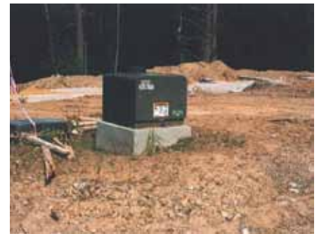
Padmount located in remote area. Outside case was energized!
